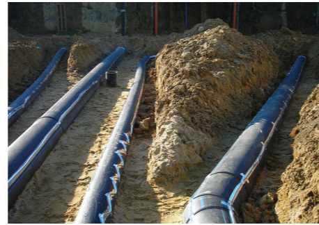
Pipeline in Strzelce Opolskie, Poland
